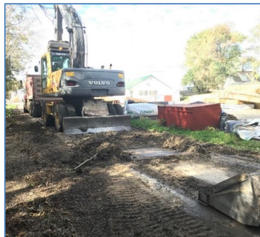
3. Equipment used to clean up and remove windrowed organic material: skid steer (bucket shown in the lower right), a small rubber tired backhoe, and a tri-axle dump truck.
