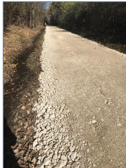
4. After re-surfacing with a 6-inches compacted course of 3-inch minus stone laid on the regraded trail. The original trail screenings below were still white and clean.
